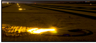
In-Pavement Runway Guard Light
