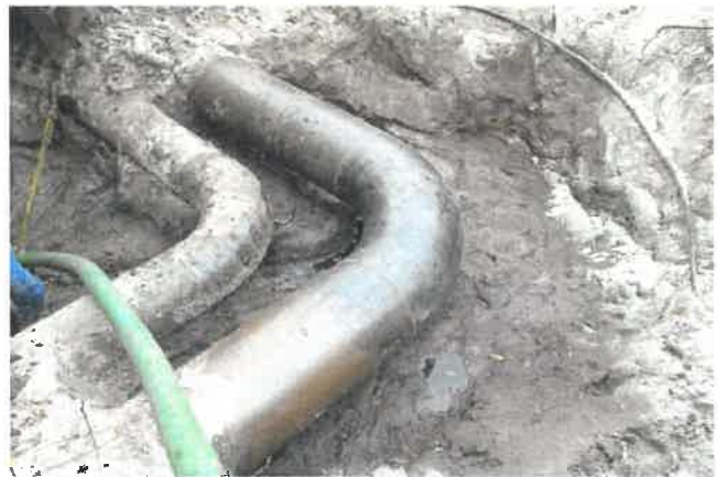
18-inch Piping View
