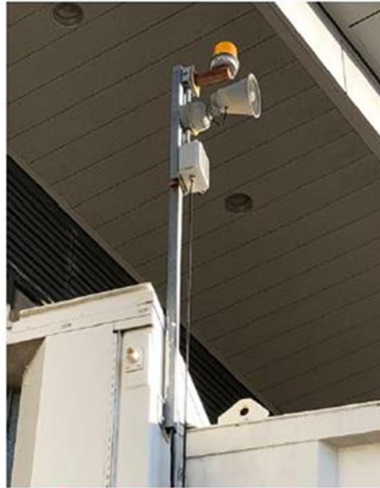
Horn & Beacon (exterior)
