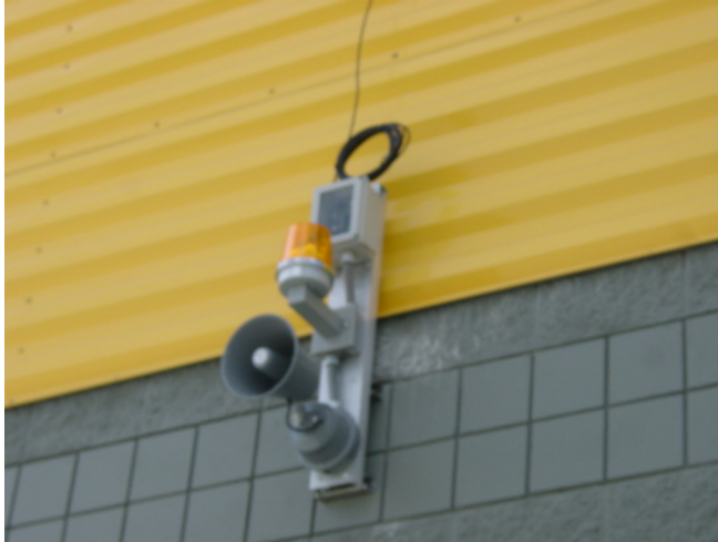
Exterior Remote Enunciator unit
